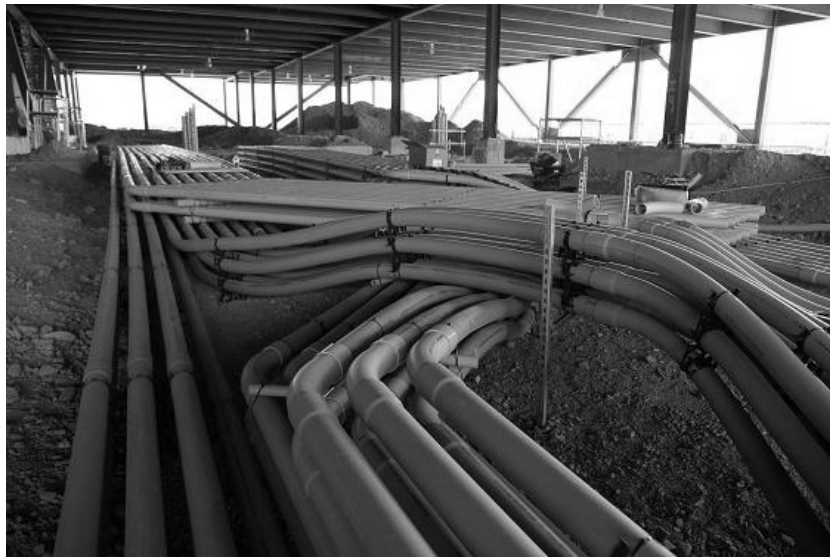
Figure 1.1: Underground Electrical Conduit in Data Center Construction
